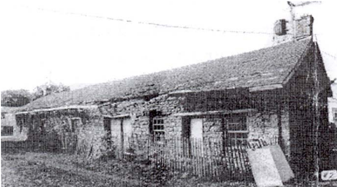
Here is how the building looked before the Museum Foundation took it over.
